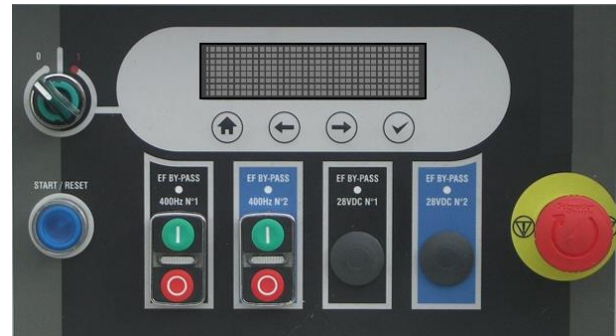
Control panel for D2 design
