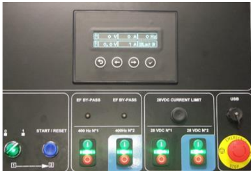
Control panel for D1 design
